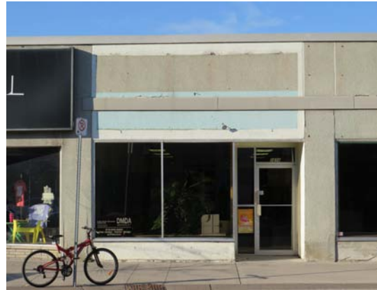
Figure 155. A traditional Main Street building façade that is covered with non-traditional materials and is missing signage
