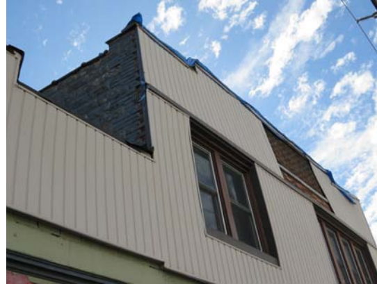
Figure 124. Example of where original building materials have been covered up
