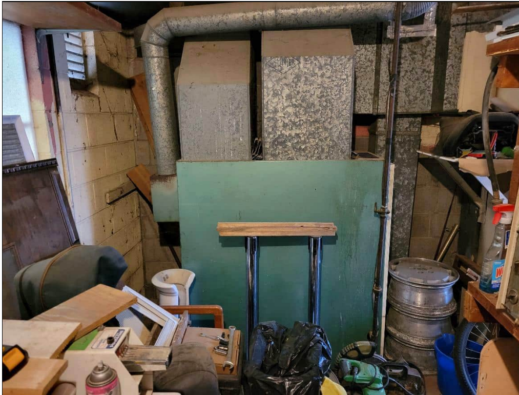
Photo 9: The mechanical room, including the furnace as well as clutter and debris.
