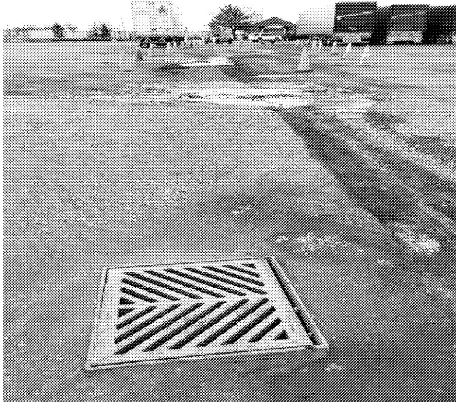
Photograph 5: catch basin outside limits of loss location (02/09/19)
