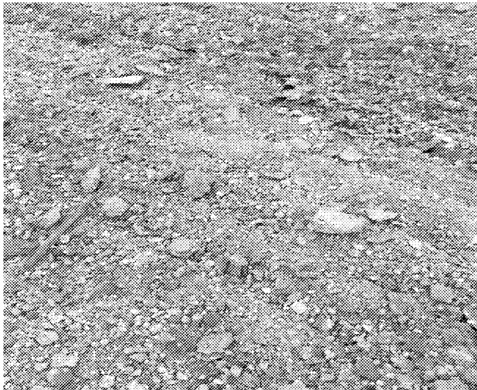
Photograph 10: debris found in the original parking lot material (exposed during excavation) (02/10/19)
