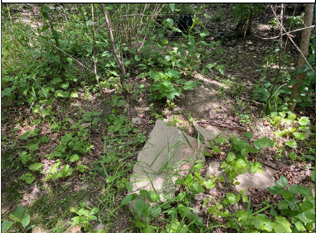
17. Partially buried concrete debris.
