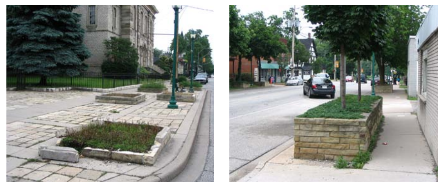
(Left) A damaged planter in front of Mackenzie Hall requiring repair. (Right) An example of a taller planter that should be lowered to a height consistent with other planters throughout the commercial area.
