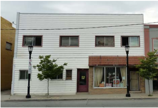
Vinylcide – this building is clad in sundamaged and degraded vinyl siding.
