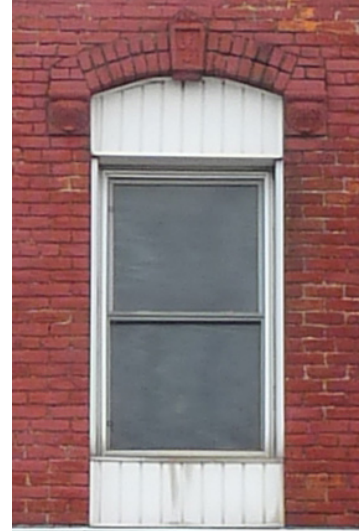
This window is reduced to a third of its useable area.
