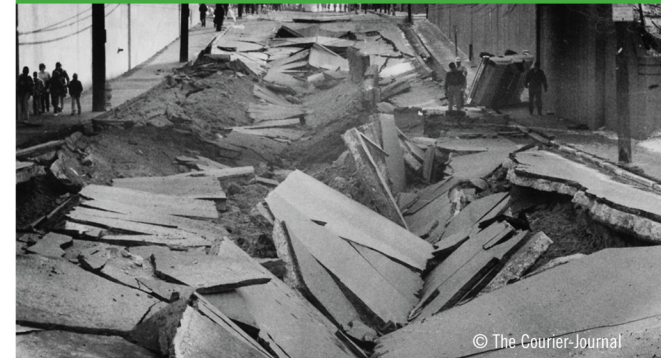
A sewer explosion in 1981, blamed on an illegal release of the solvent hexane, destroyed two miles of Louisville streets. It took nearly two years to repair the sewer lines and several more months to finish street repairs.
