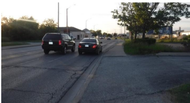
Photo 4: Deficient westbound lane width
