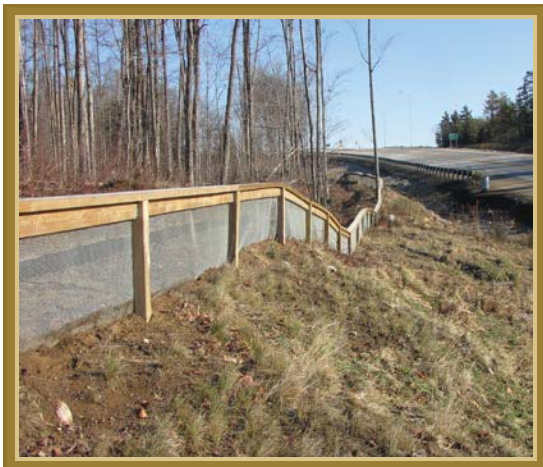
Figure 4: A wire mesh fence installed on a grassy embankment next to a road. The fence is designed to prevent animals from crossing the road. M
