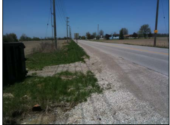
Plate 4: County Road 17 facing north, note disturbance due to ditching up to property line.
