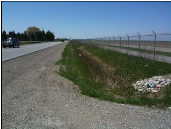
Plate 14: County Road 42 facing west, note disturbance due to ditching up to property line.
