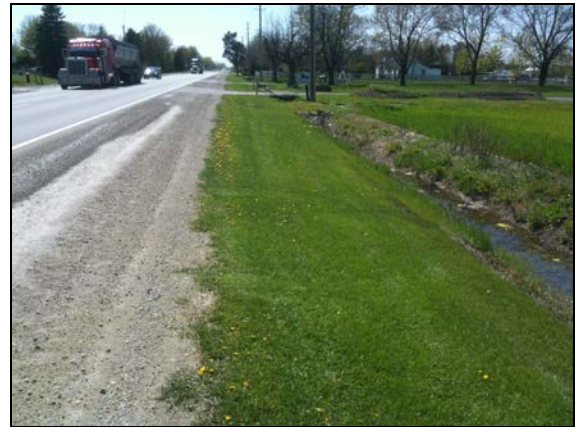
Plate 29: County Road 42 facing west, note disturbance due to ditching up to property line.
