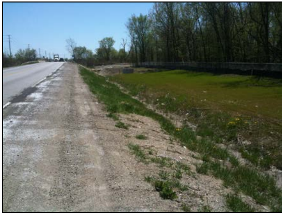
Plate 13: Lauzon Parkway facing south, note disturbance due to sanitary sewer construction ditching and stripping up to property line.
