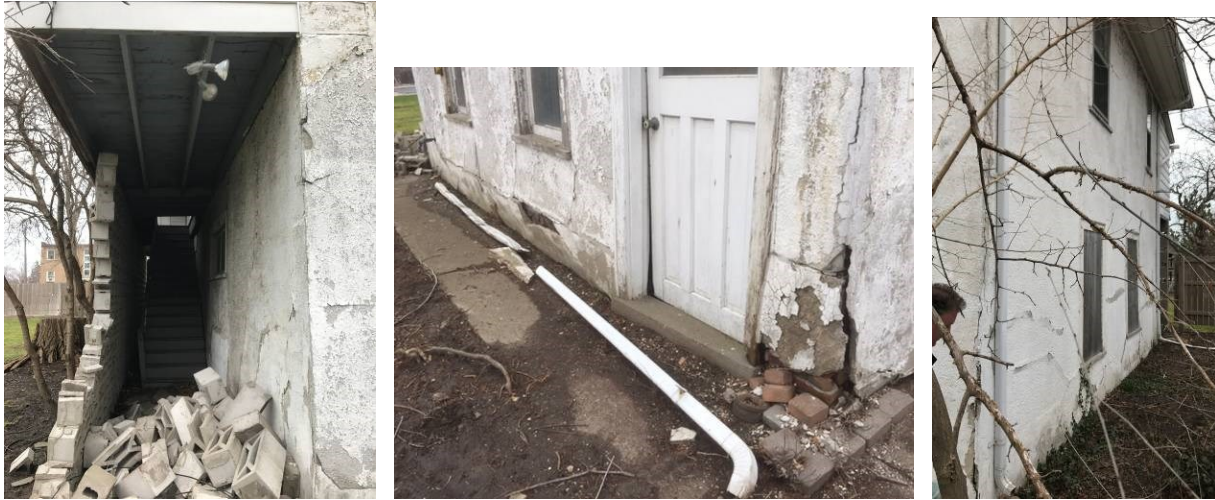
Deteriorated locations, garage, 6425 Riverside Drive East (2017)
